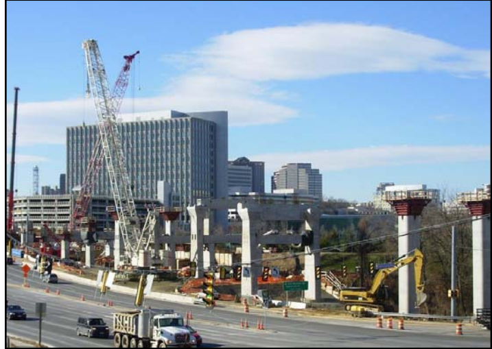
Construction of the Tysons East Station at Route 123 and Coleshire Road (Capital One Headquarters in background).
