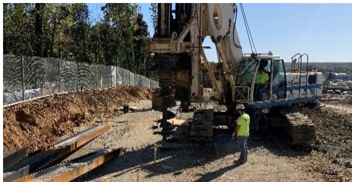
From Top to Bottom: Rendering of the Residences at North Hill Development; Site clearing and grading is underway (Richmond Highway is on the right); Drilling/installation of soldier piles for the retaining wall.
