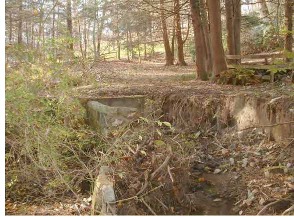
Photo 3.27 Erosion located between Old Dominion Drive and Georgetown Pike (DFDF011.E001).
