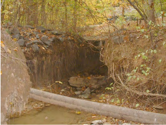
Photo 3.56 An 18-inch outfall causing severe erosion located downstream of the outfall shown in Photo 4.1 (DFSB006.P005).
