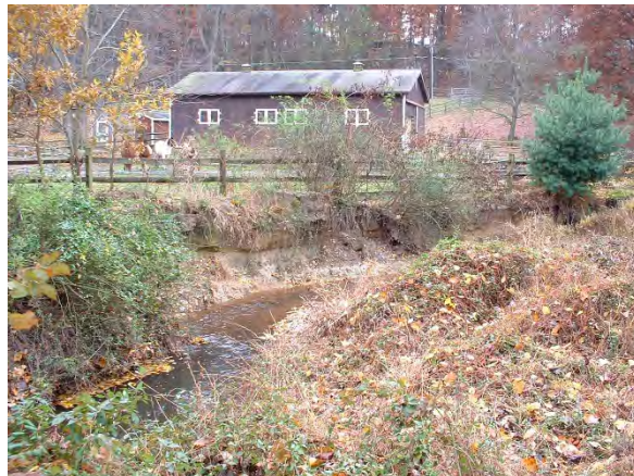
Photo 3.97 Erosion located on the mainstem of Little Difficult Run, directly east of Colt Run Road in the Roan Stallion Estates subdivision (DFLD013.E001).
