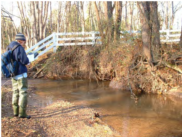
Photo 3.12 Erosion just south of Eisenhower Lane (DFPR005.E001).
