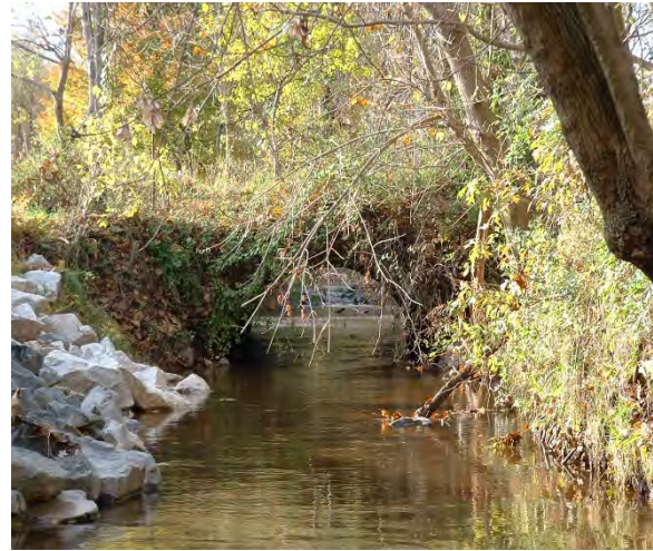
Photo 3.25 Upstream and downstream bank erosion at Leesburg Pike (DFCR001.C001).
