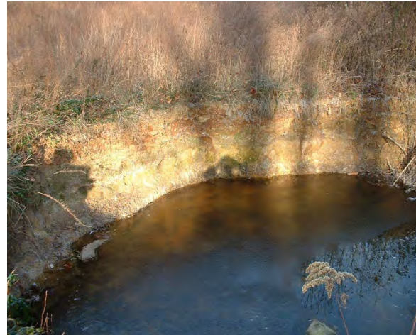
Photo 3.10 Erosion located near confluence of Dog Run with Piney Run (DFDG001.E001).
