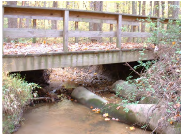
Photo 3.65 Wooden bridge where stream flow is causing moderate erosion. Located just west of Steeplechase Drive (DFGL008.C001).
