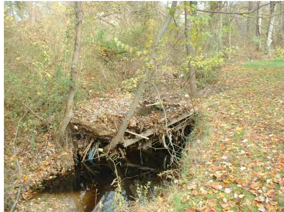
Photo 3.79 A severe obstruction located upstream of Chain Bridge Road near Echols Street (DFWC028.T001).
