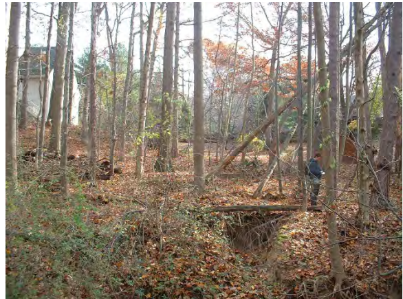
Photo 3.23 Erosion at outfall pipe located off of Hidden Creek Drive (DFDF020.P004).
