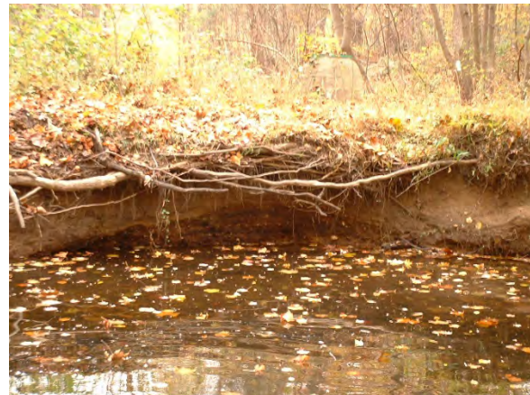
Photo 3.51 Obstruction upstream of Lake Fairfax located near Park Overlook Drive (DFCR015.T001).
