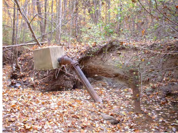
Photo 3.57 Pipe located south of Sunrise Valley Drive and just east of Barton Hill Road. Major erosion around the structure is evident (DFSB006.P003).
