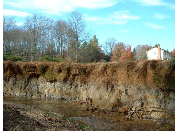
Photo 3.119 Heavily eroding bank on the South Fork Run mainstem, directly north of the intersection with Fox Mill Road and Deerfield Drive (DFSF007.E001).
