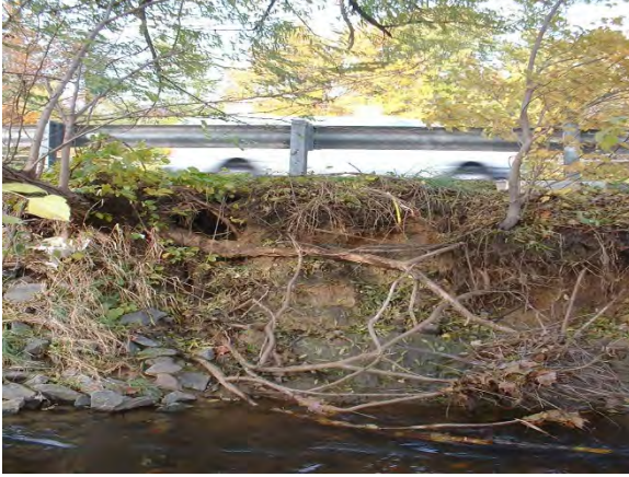
Photo 3.26 Severe erosion that could pose a threat to road safety along Route 7 to the east of Carpers Farm Way (DFCR001.E001).
