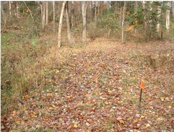
Photo 3.5 Earthen berm located in the upper reaches of Captain Hickory Run near Thunderhill Court (DFCH009.T001)
