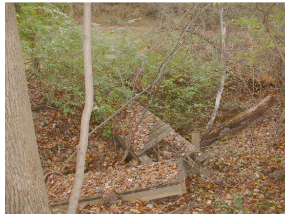
Photo 3.112 Obstruction located just south of East Hunter Valley Road (DFAB002.T002)
