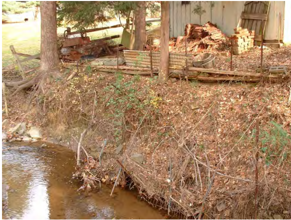
Photo 3.3 Erosion on the right bank of Captain Hickory Run near the end of Constellation Drive (DFCH010.E001)
