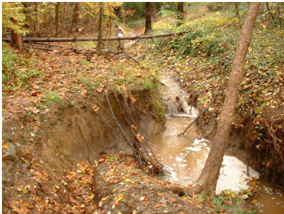
Photo 3.46 Erosion located on a tributary to Colvin Run between Buttermilk Lane and Hunt Club Road (DFCR012.E002)
