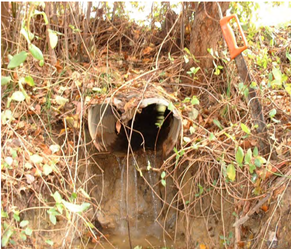
Photo 3.1 Erosion at the end of stormwater pipe located off of Collin Farm Land (DFCH021.P003).
