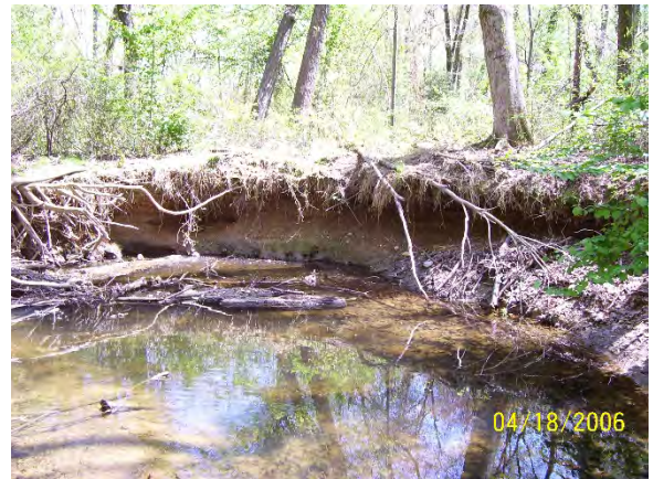
Photo 3.59 Erosion located between Old Trail Drive and Millenium Lane (DFSB015.E001).
