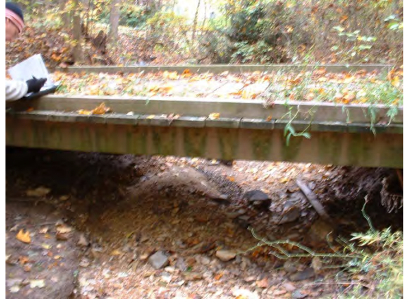
Photo 3.64 Wooden bridge where stream flow is causing moderate erosion. Located just off of Bassett Lane (DFGL008.C004).
