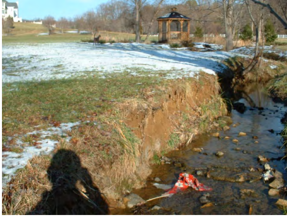
Photo 3.124 Erosion point on the west side of Hunter Mill Road at the intersection with Conejo Land (DFRB012.E001).
