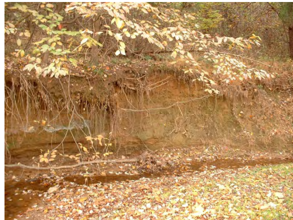
Photo 3.47 Erosion located on reach just west of Hunter Mill Road near Little Run Farm Court (DFCR008.E001)
