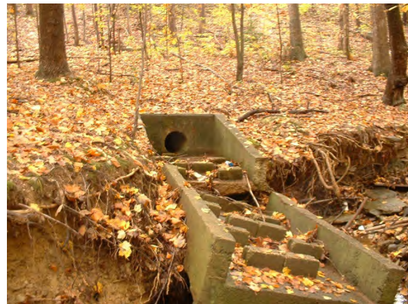
Photo 3.45 Erosion at a 12-inch outfall located just south of North Shore Drive (DFCR013.P003).
