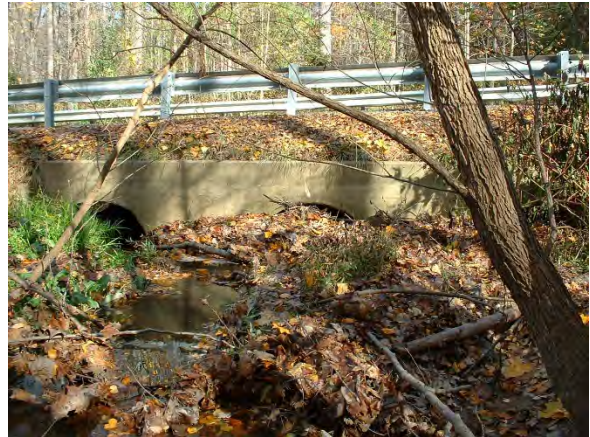
Photo 3.94 Crossing under Fox Mill Road north of Shady Mill Lane. Crossing has excessive sedimentation (DFLD015.C002).
