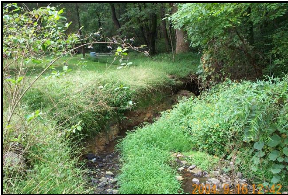
3' eroded bank with no buffer.
